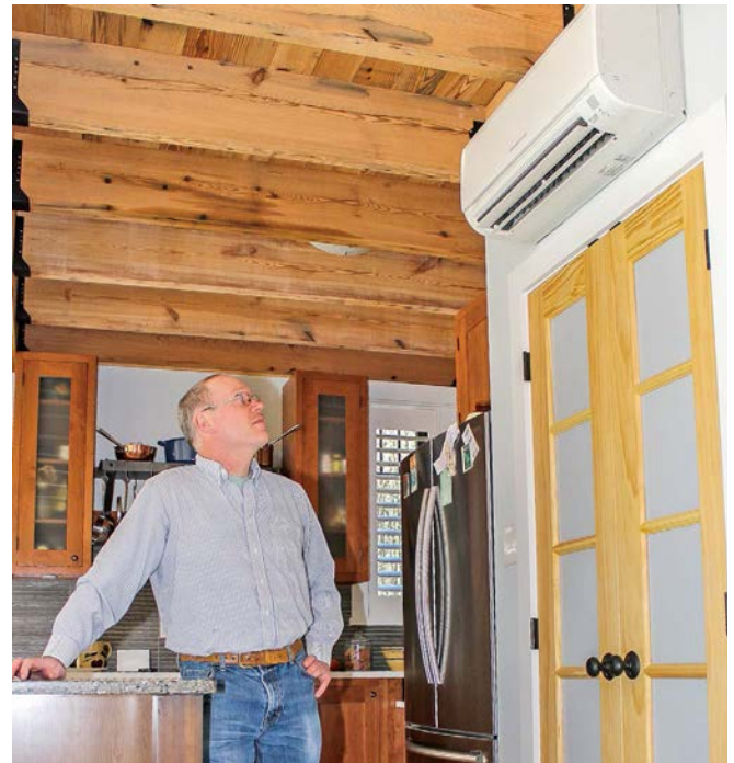
Sean checks out the minisplit multizone heat pump, which provides auxiliary cooling during the hottest part of summer.
